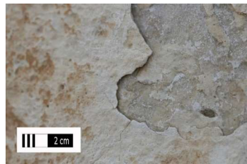
Figure 4. 2. 15 Discolouration with orange together with scaling part and salt sub-efflorescence
