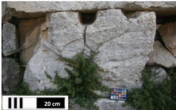
Figure 4. 2. 18 A star crack
