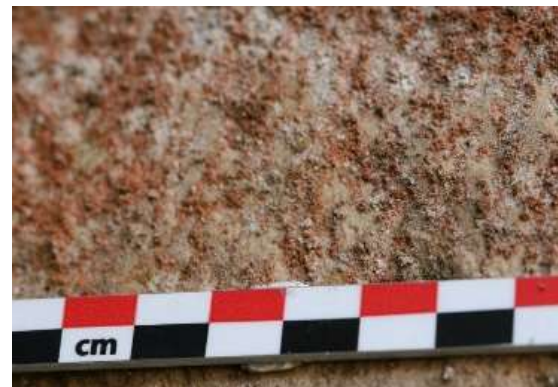
Figure 4. 2. 8 The microorganism colonization on the second pillar from west of the first northern row of Pillar of Building (4) (east face)
