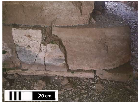
Figure 4. 2. 22 Splitting in Building (35)
