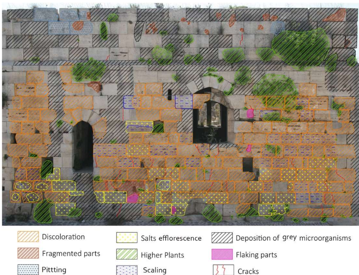
Figure 4. 3. 28 The deterioration mapping of the external east facade of the building (36)
