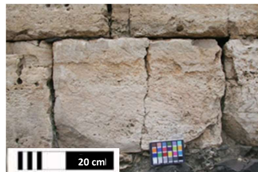
Figure 4. 2. 17 A fracture in the middle of the stone
