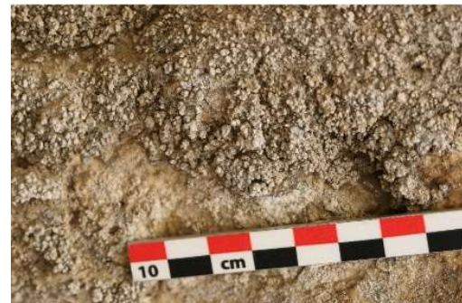
Figure 4. 2. 24 Framboidal encrustation case in Building (38)
