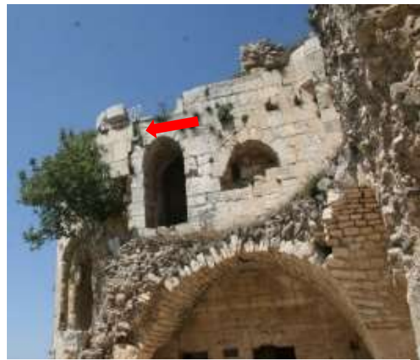
Figure 4. 2. 10 shrub that grows on the east corner of Building (39). The red arrow refers to massive crack caused by the plant
