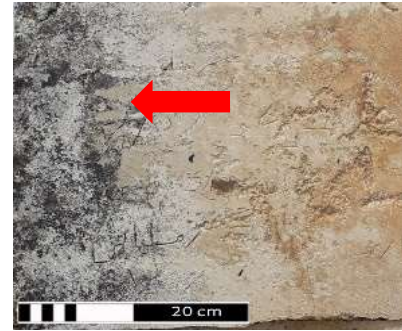
Figure 4. 2. 9 Black and white microorganism colonization on the outermost west edge of the south external façade of Building (46)
