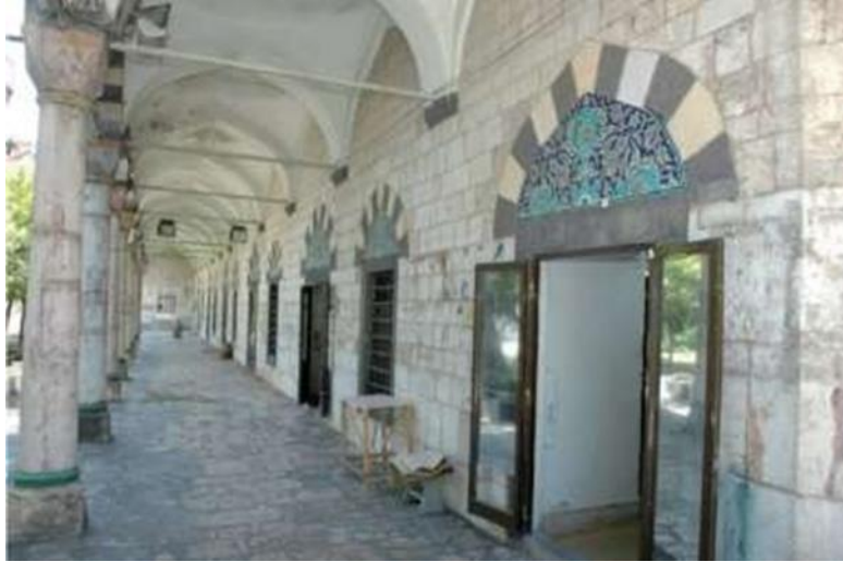
Figure 29 The portico of the tabhane in the west of the mosque (Güçhan & Kuleli 2018: 12)
