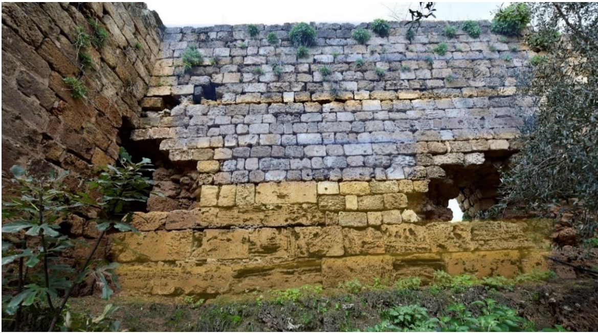
Fig. 54- Junction of wall 18 and tower 19 on the eastern façade of the enclosure.
