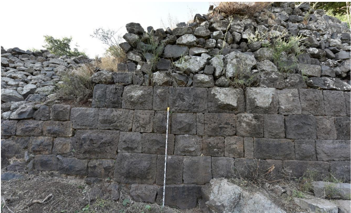
Fig. 90-Foundations of the southern castle wall constructed from Roman period spolia. (B. Major).
