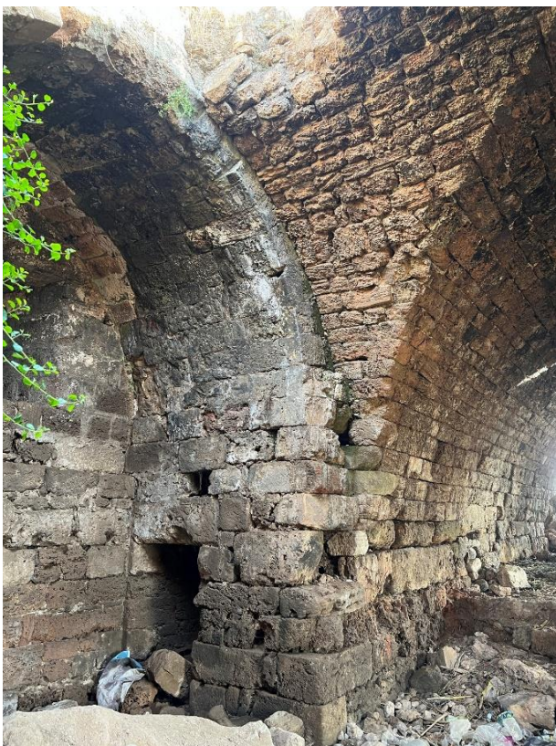
Fig. 23-Junction in between the tower 4.o and the space 3.o the vault was added later.
