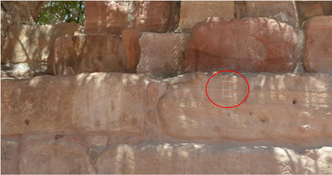
Plate 65: A minor act of Graffiti vandalism at the site. (Photo Taken by the Author 2022)
